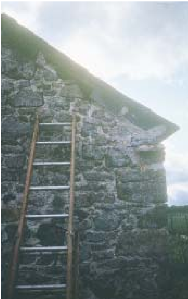
Picture 8 When checking a site for potential nest cavities don't overlook the outside of the building. Note the white lines on the wall to the right of the ladder. David Ramsden
