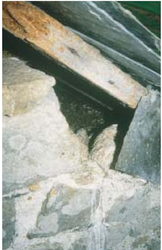
Picture 9 This cavity (note the debris and droppings) was accessible only from the outside of the site and could easily have been missed during a survey. David Ramsden
